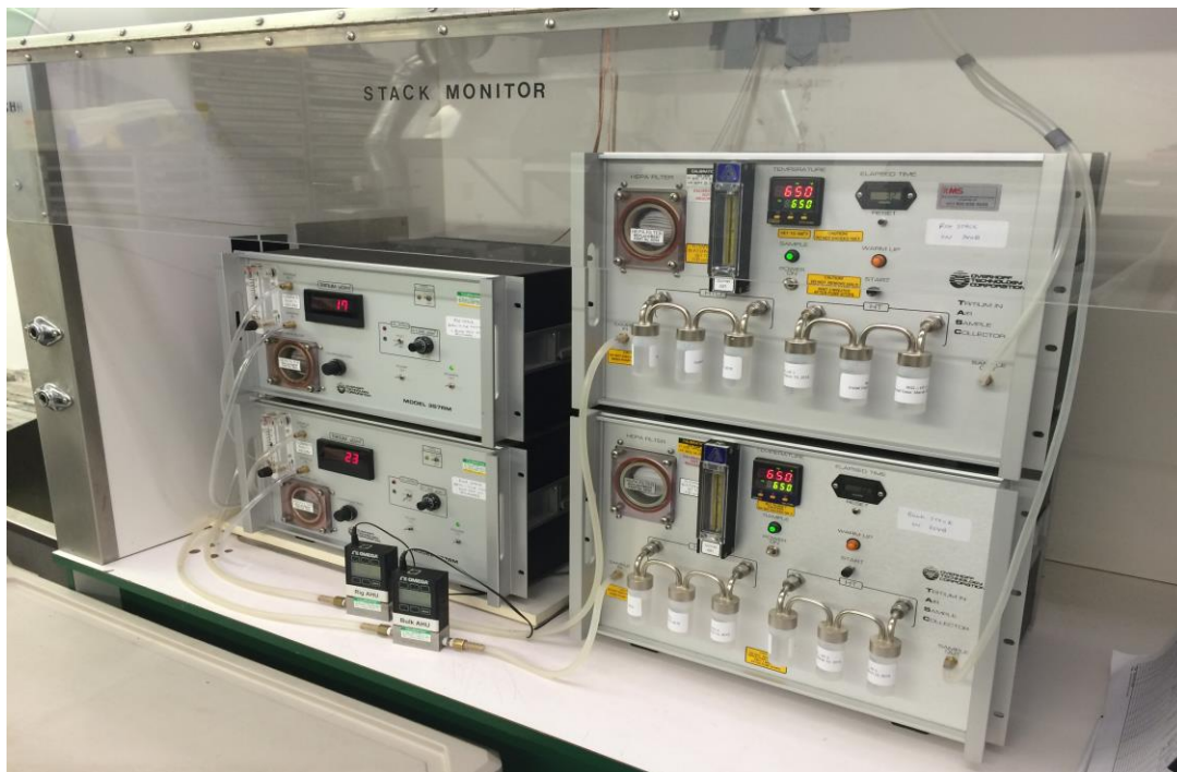
FIGURE 10: STACK MONITORING EQUIPMENT
