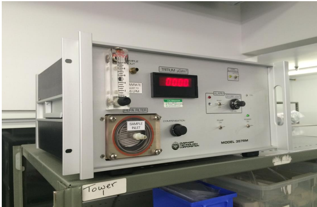
FIGURE 9: TRITIUM-IN-AIR MONITOR IN ZONE 2
